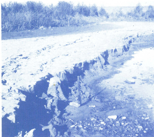
Figure 3. Lateral spread cracks and caved stream banks resulting from liquefaction along the Virgin River near St. George. Photo by W.E. Mulvey, UGS.
