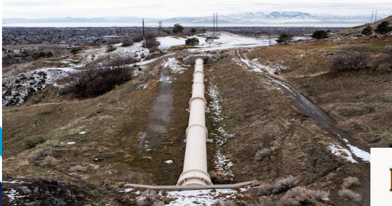
A section of the Alpine Aqueduct runs above ground where it crosses a fault in the hills above Orem on Thursday, Jan. 6, 2022. | Spenser Heaps, Deseret News | Purchase Photo
