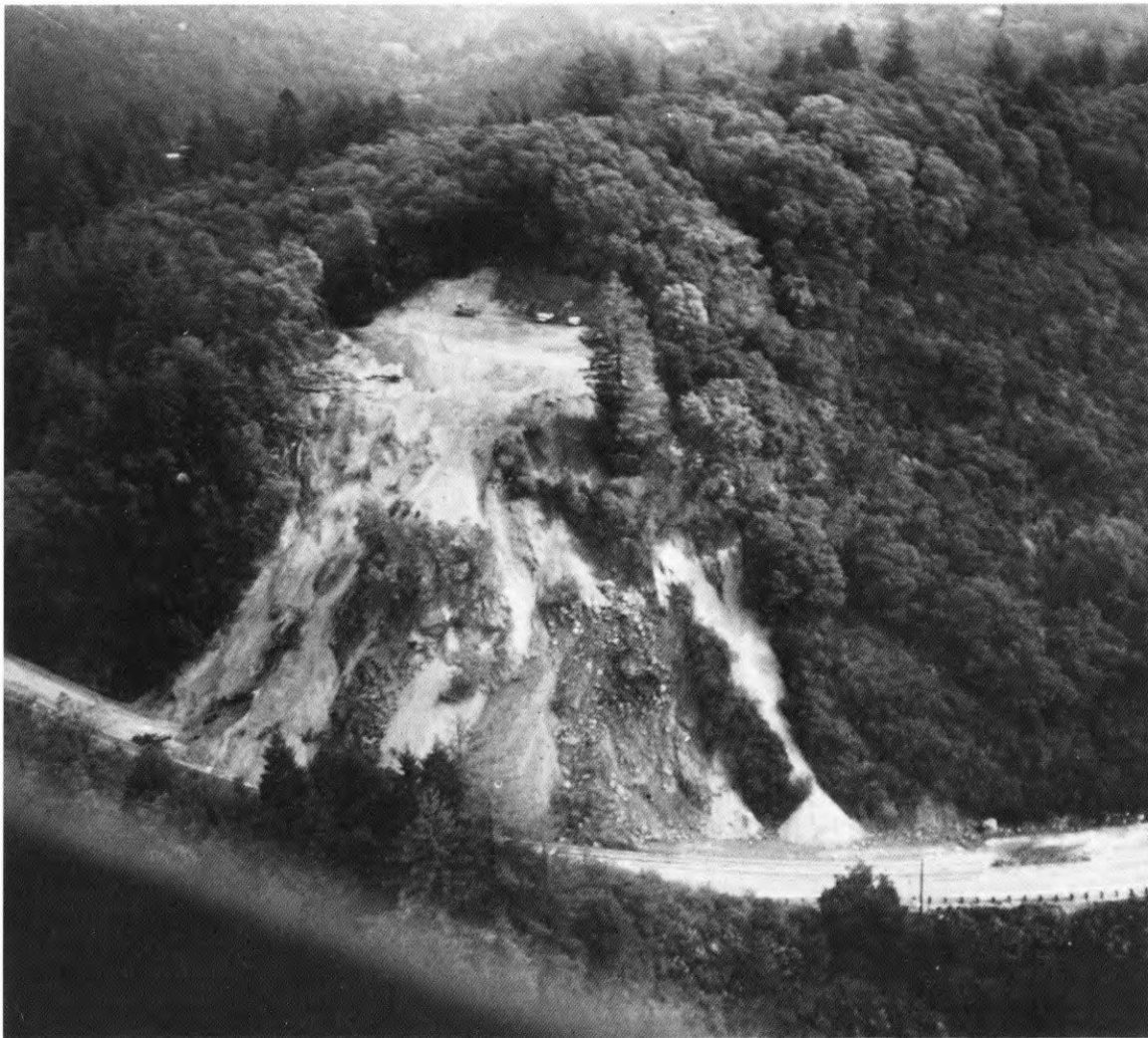
Figure 20. Aerial photograph of rock slide near summit of Santa Cruz Mountains that has an estimated volume of 6,000 to 10,000 cubic yards. Slide nearly completely blocked northbound lanes of Highway 17 that links Santa Cruz and surrounding
