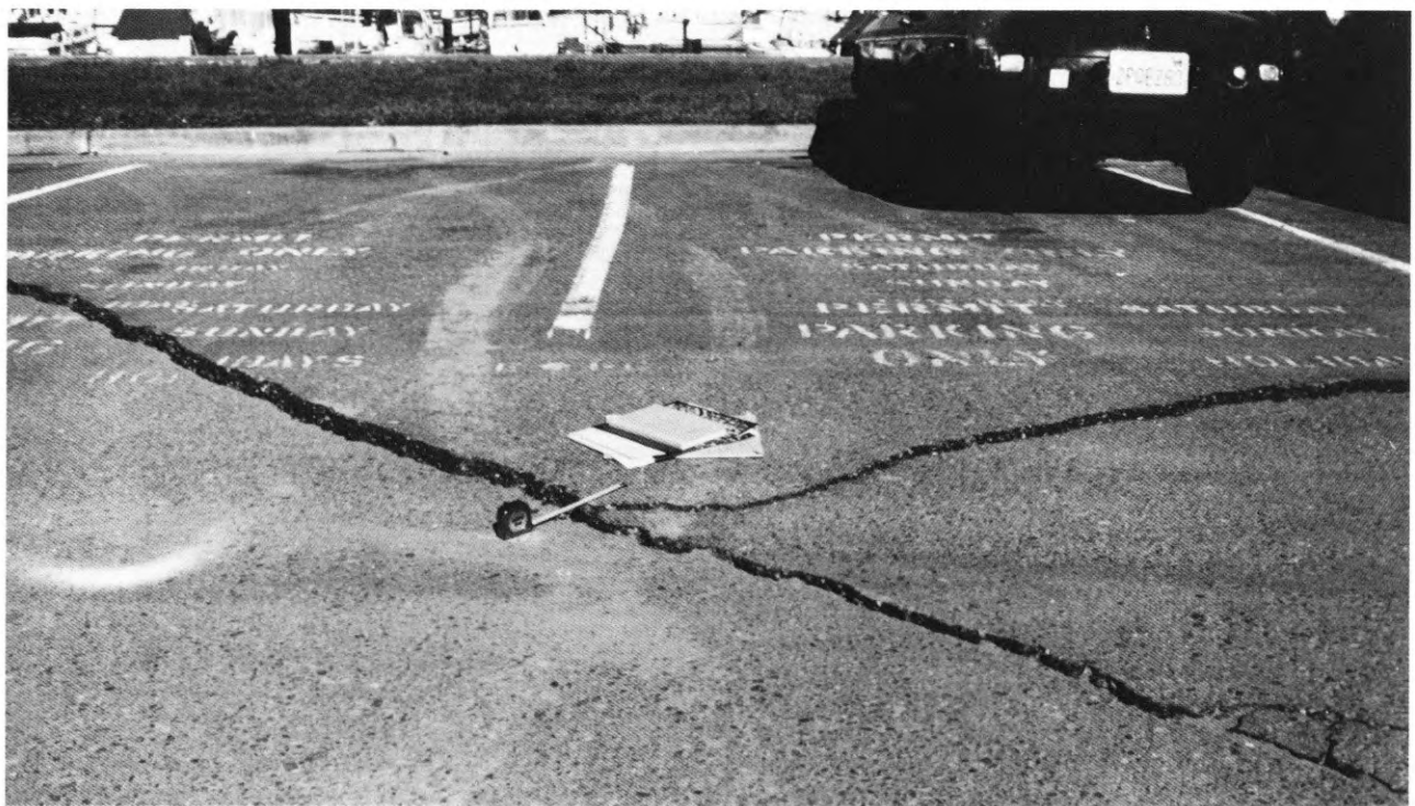
Figure 25. Extension cracks in Marina district formed by lateral spreading of liquefied sandy landfill.
