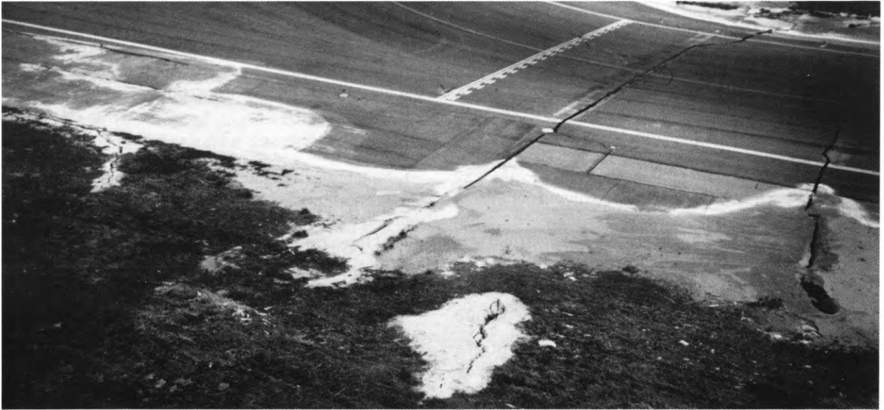
Figure 28. Sand boils at Oakland International Airport.
