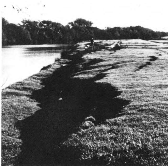
Figure 23. Lateral spreading along Pajaro River banks due to liquefaction.
