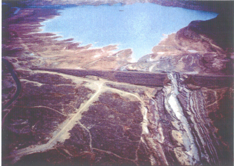
Figure 7. View looking north at the Quail Creek south dam failure, January 1989. Photo courtesy of Benjamin Everitt.
