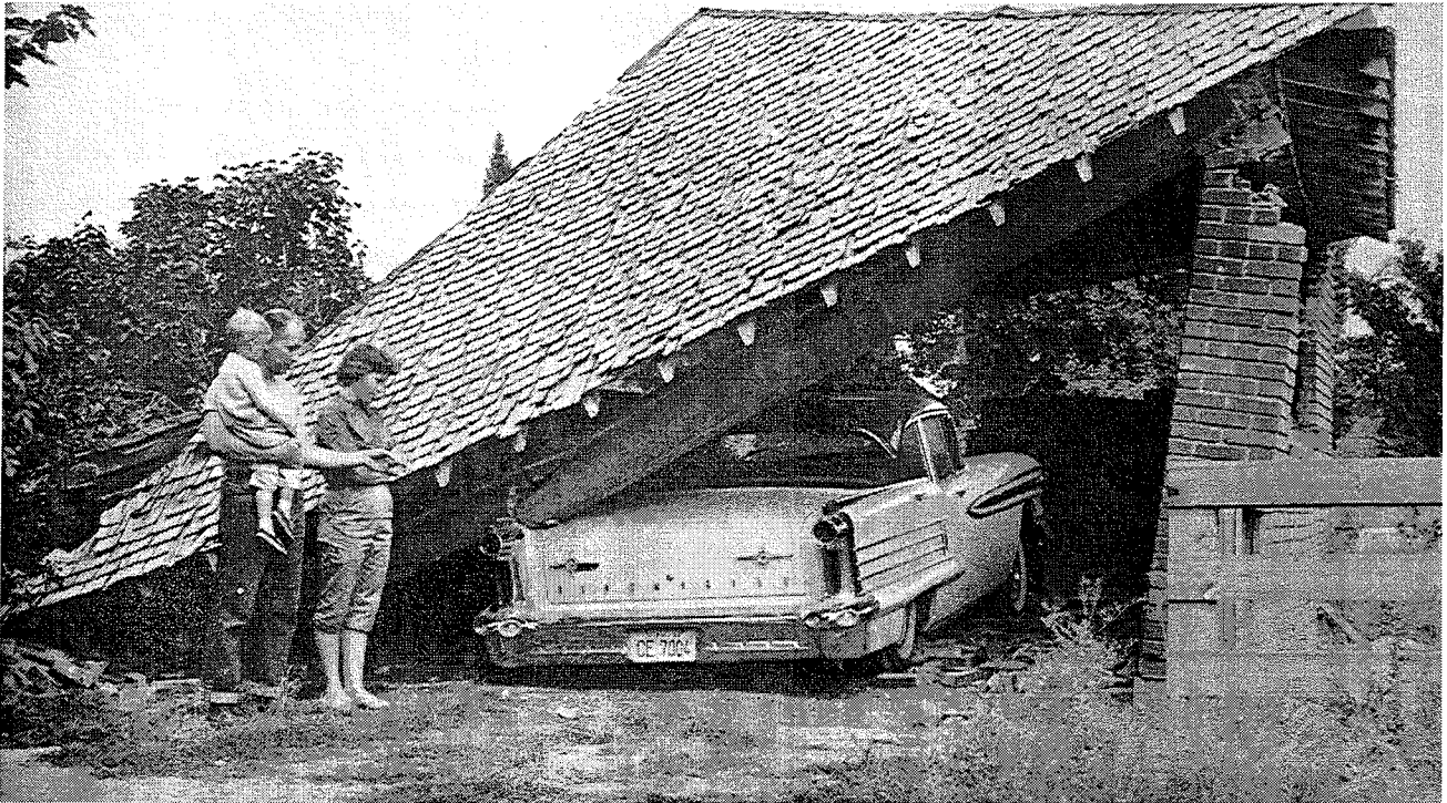
Figure 9: URM pier failure.
