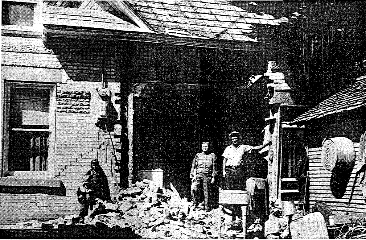
Figure 6: URM wall collapse from earthquake damage.
