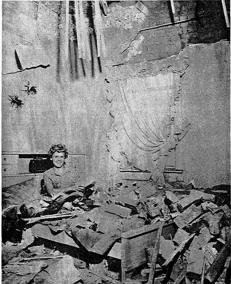
Figure 4: Interior URM wall collapse.
